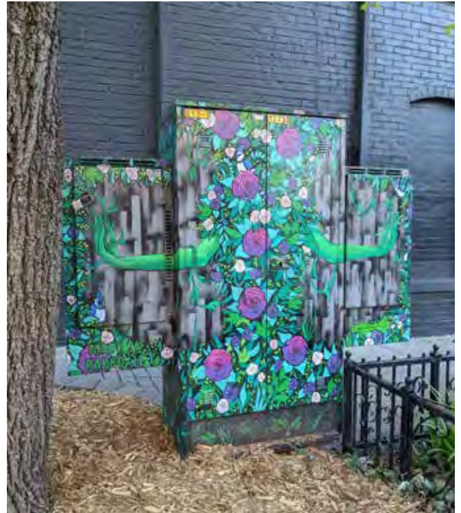
Figure 91: A painted utility box on Elm Grove Avenue near Queen Street West.
