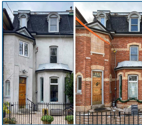
Heritage Grant Program | Funding support for masonry restoration was awarded to this property in the Cabbagetown Northwest Heritage Conservation District. Before conservation (left) and after conservation (right).
