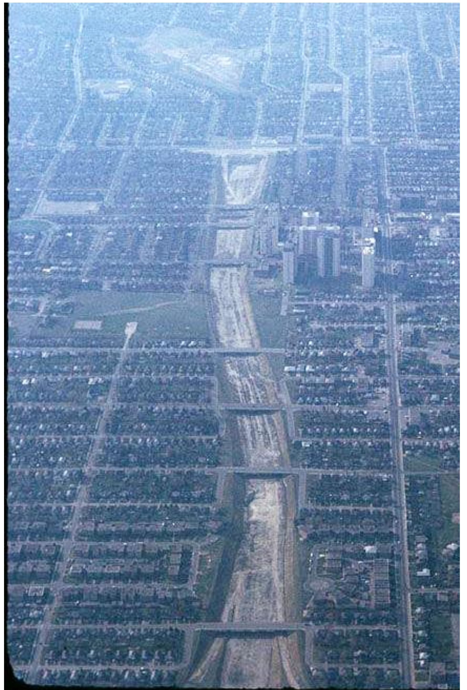
A view of Allen Road under construction between Lawrence Ave W and Eglinton Ave W in 1974.
